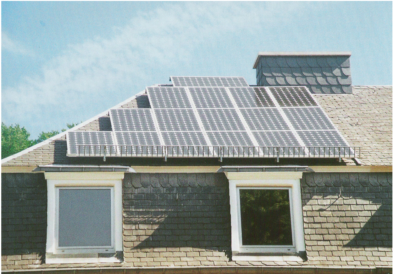
Abb.: 2,8-kWp-Photovoltaik-Anlage (Foto: S. Brocker)
